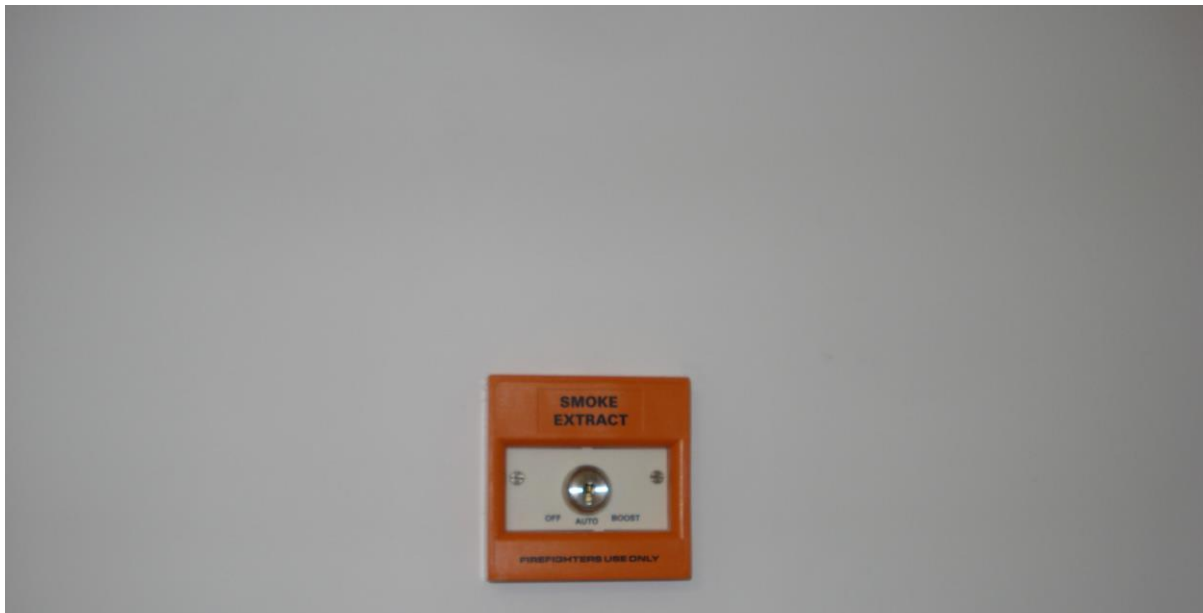
Fireman's Override Key-Switch. One on every appropriate Staircase Landing. OFF which disables the complete Smoke Flushing System. AUTO which is the normal default position. BOOST which makes the Smoke Flushing System run at full speed / extract rate.
